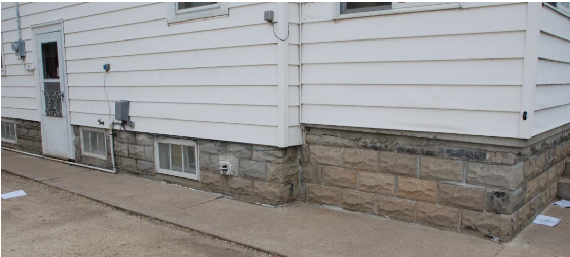
Photographs: 411 2nd St SW, detail of foundation, looking northwest and garage, looking northeast, 4/7/2014, Andrew Bell, Svendsen Tyler, photographer.
