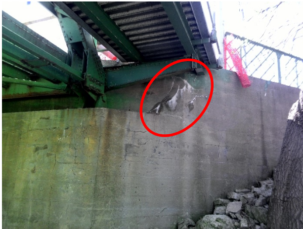
South Abut. Back Wall – Major cracking w/ efflorescence
