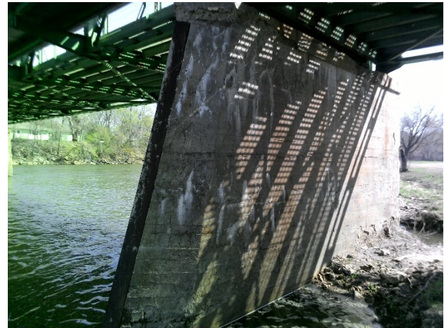
S. Pier, West End – Major cracking w/ efflorescence
