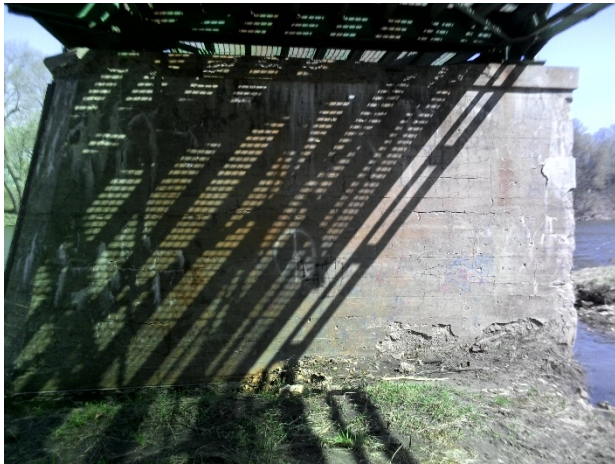
S. Pier, S. Wall – Delamination, spalling, cracking w/leaching
