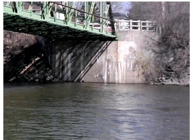
North Abutment – Major cracking w/ efflorescence
