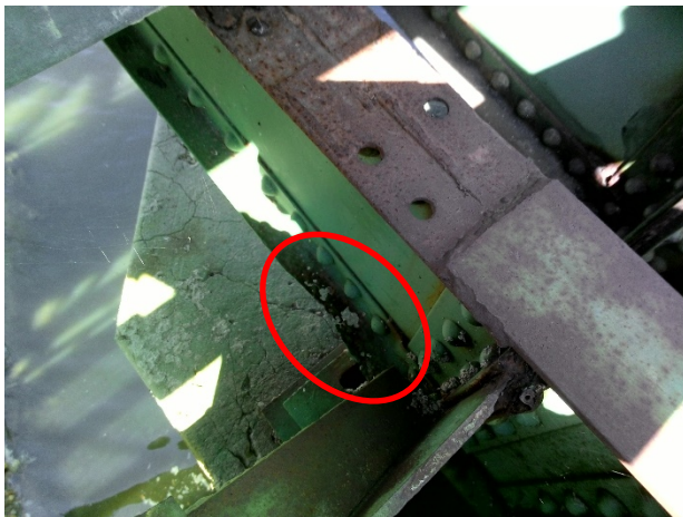
Sidewalk Bracket @ S. Pier – Section loss through bott. flange
