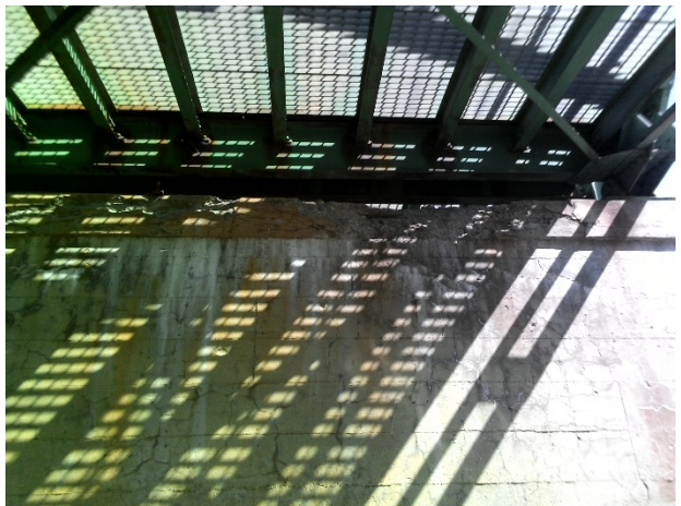
S. Pier Cap – Major delamination, crushing. Loss of bearing
