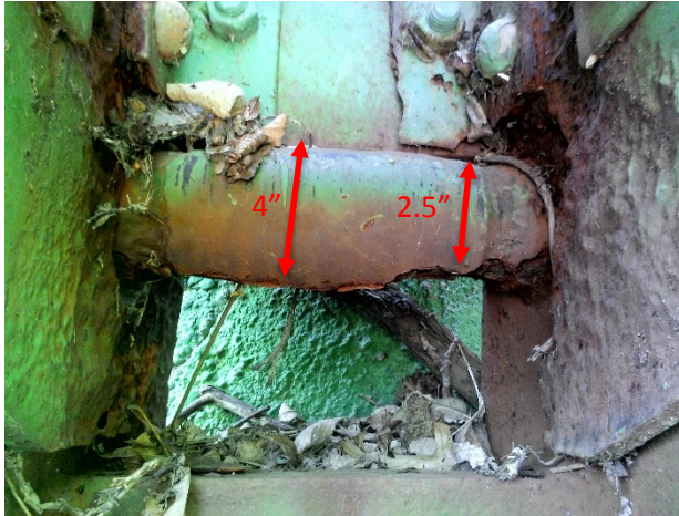
Southwest Bearing at South Abut. – Major section loss
