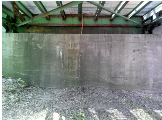
South Abut. – Large cracks, spalling w/ exposed rebar
