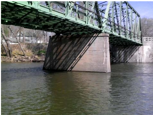
North Pier, South Wall – Cracking w/ efflorescence
