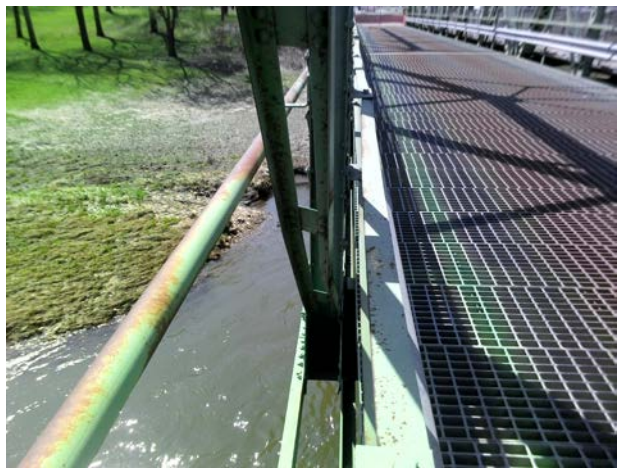
West Truss, U2L3 – Distortion, out of plane bending
