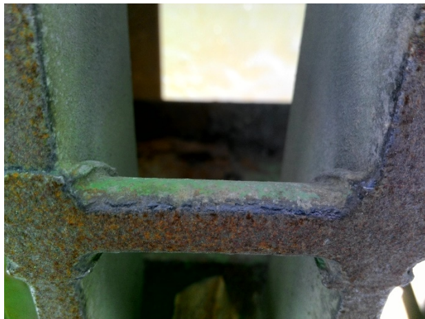
Typical corrosion on deck grating
