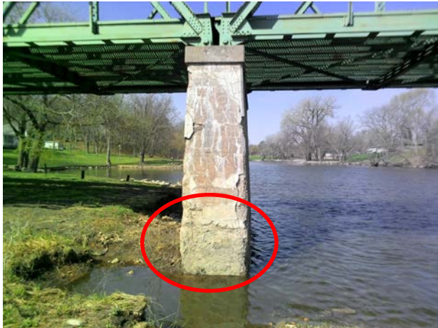
S. Pier, East End – Major spalling near waterline
