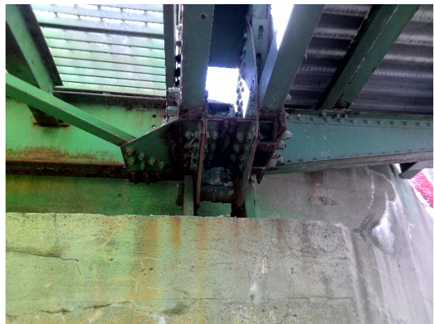
South Abut. Seat – Major cracking w/ efflorescence
