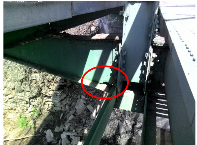
S.W. Bracket @ N. Span, 4 th Panel – Section loss through bott. Flange
