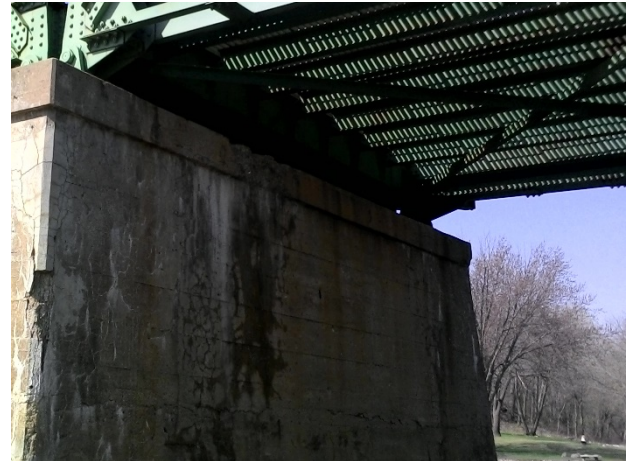
S. Pier, N. Wall – Major cracking w/ efflorescence
